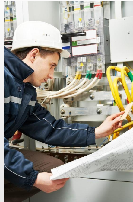
Service and Revamping
